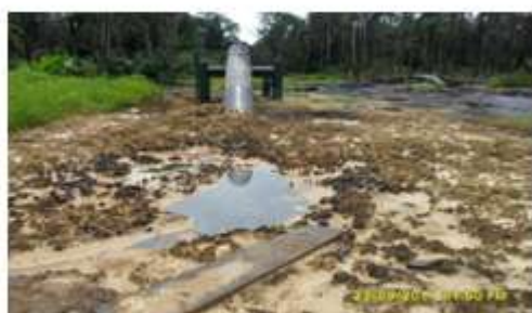
Fig 3: Part of spill impact at 20" Kolocreek-Rumuekpe Pipeline right of way at Ogbogoro (SPDC 2011).
