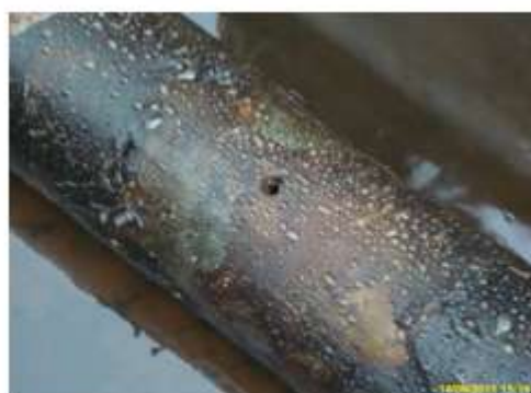
Fig 2: Spill due to drilled hole on a flow pipeline in the Niger Delta
