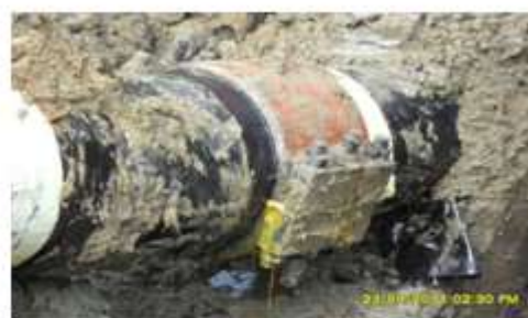
Fig 4: Spill due to failed clamp on 20" Kolocreek-Rumuekpe Pipeline right of way at Ogbogoro (SPDC 2011).
