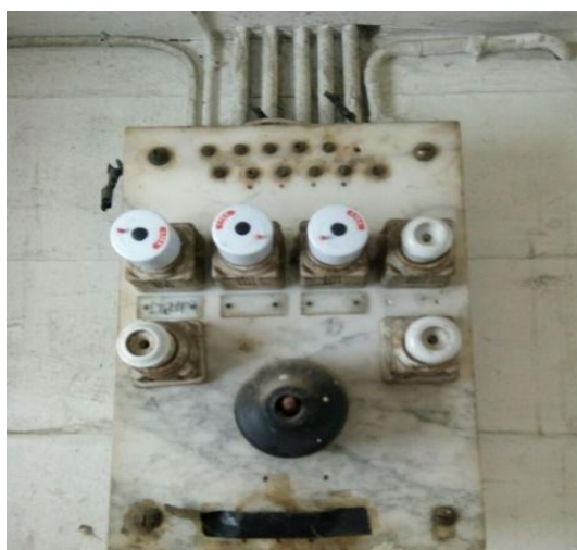
Figure 2 Electrical Panel conditions and the building of the House of Exile of Dude Karno in Laugumba village Berastagi
