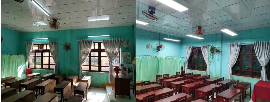
Figure 11. Classroom 1/1 of Son Phong Primary School, Hoi An (before and after installation)
